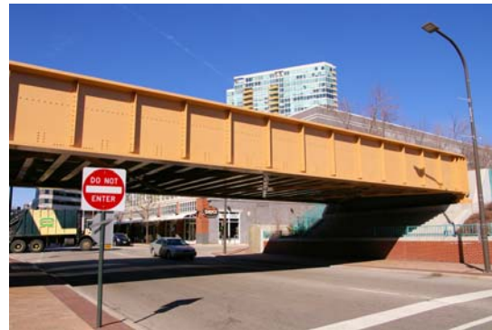
Figure 3: Rapid Transit Viaduct in Excellent Condition (Church St., Evanston, CTA Purple Line; RTA photo)
