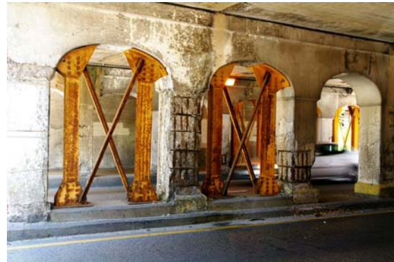
Figure 4: Rapid Transit Viaduct Beyond Useful Service Life (Hollywood Ave., Chicago, CTA Red Line; RTA photo)
